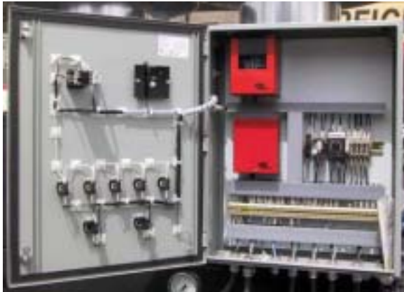
Fig 2 Burner control panel with Fireye Flame Monitor and “First-out” expansion module.
